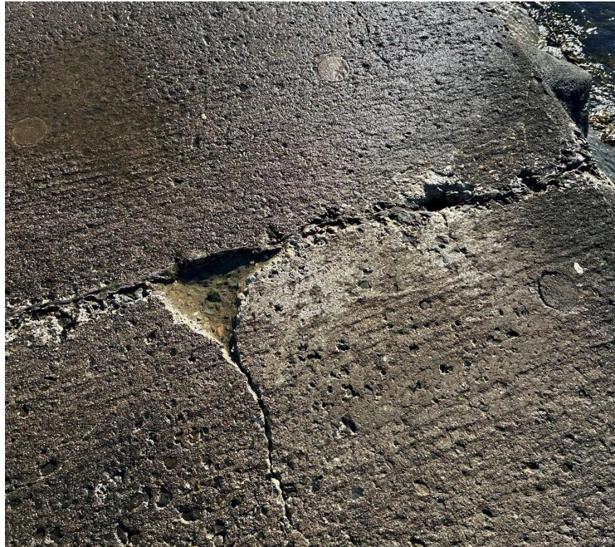
Photo 29: Sea Breeze pier concrete crack formation
