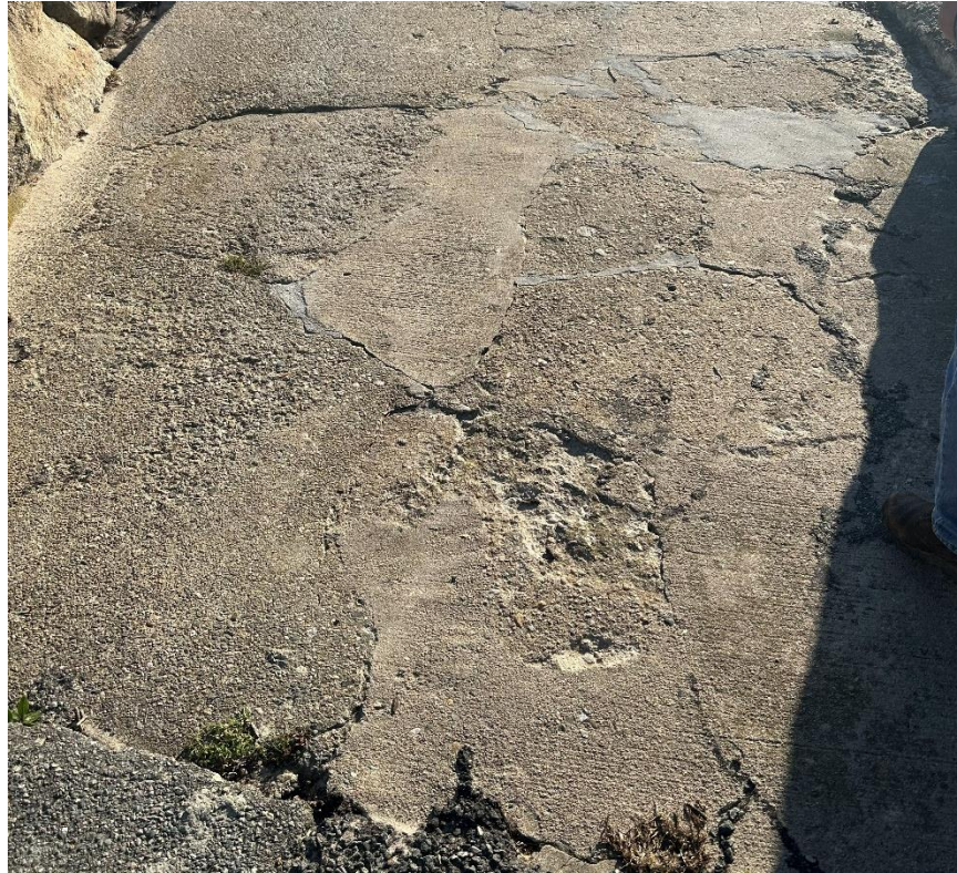
Photo 17: White Cap access way deteriorated concrete apron
