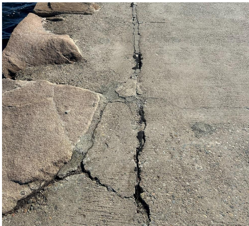
Photo 42: Osprey (South Beach) pier concrete crack formation
