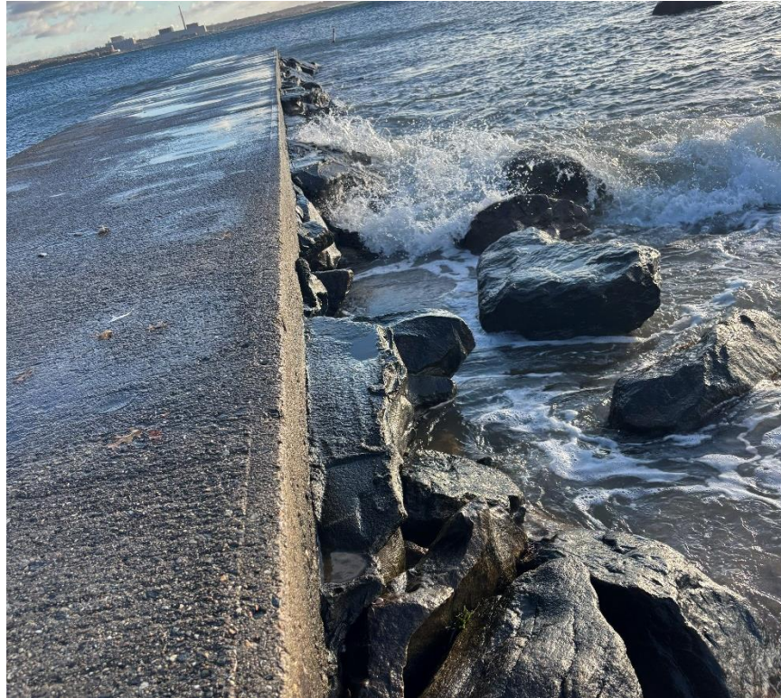
Photo 27: Sea Breeze pier South side armor stone settlement
