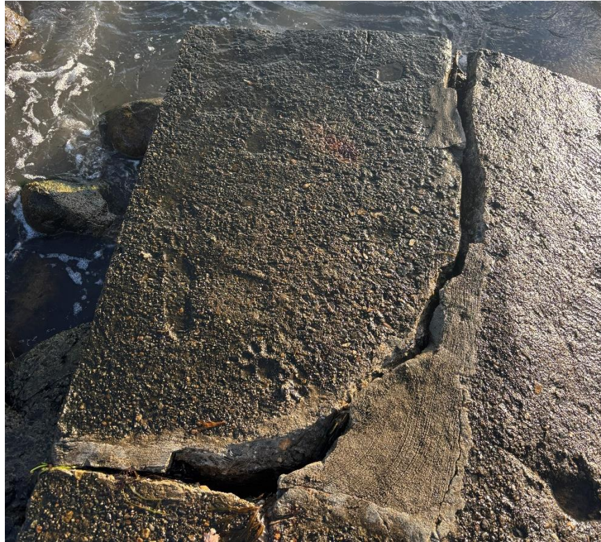
Photo 21: White Cap access way broken off encasement end
