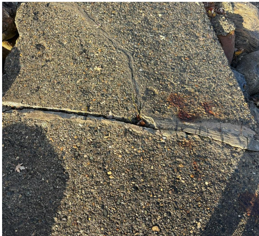
Photo 22: White Cap access way presumed pipe break location
