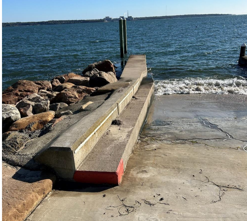
Photo 33: Sea View boat launch North wall
