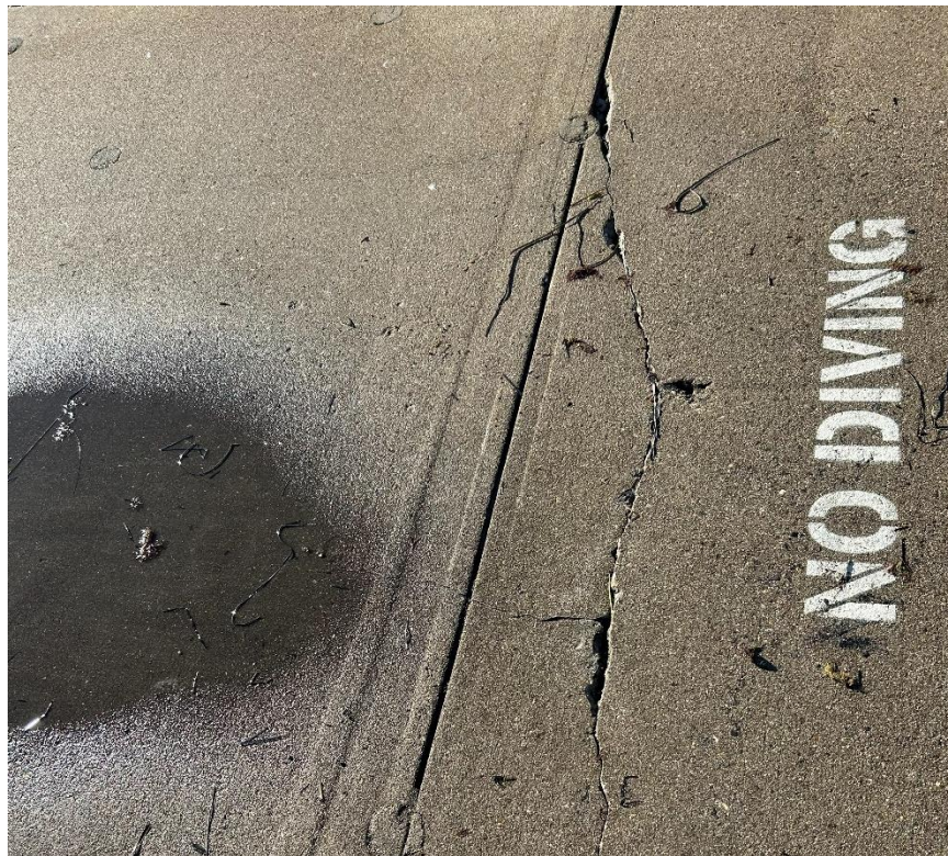
Photo 6: Nehantic pier cracked concrete
