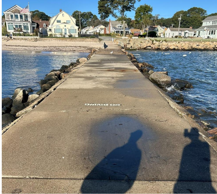
Photo 5: Nehantic pier deteriorated intermediate concrete slabs
