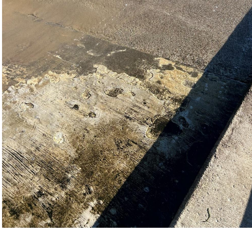
Photo 35: Sea View boat launch failed concrete overlay
