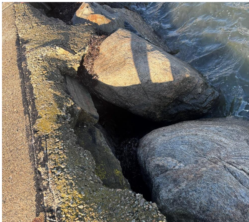
Photo 8: Nehantic pier void in stone foundation
