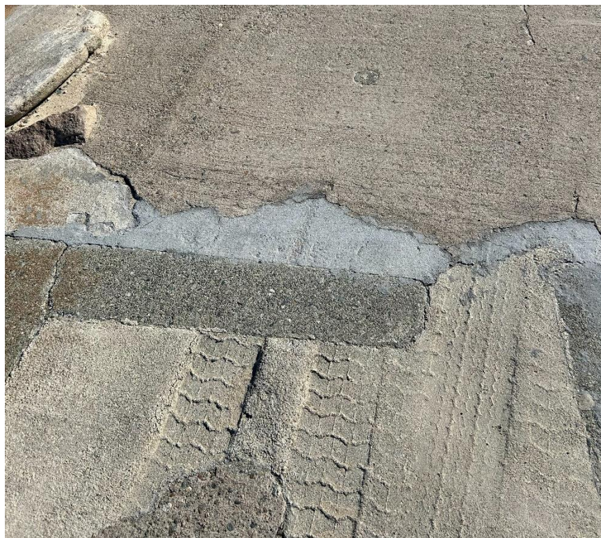
Photo 44: Osprey (South Beach) pier previous concrete crack repair
