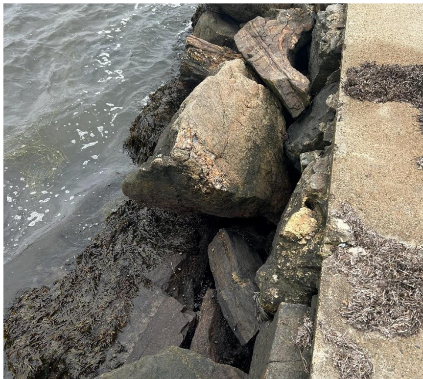
Photo 7: Nehantic pier displaced armor stone
