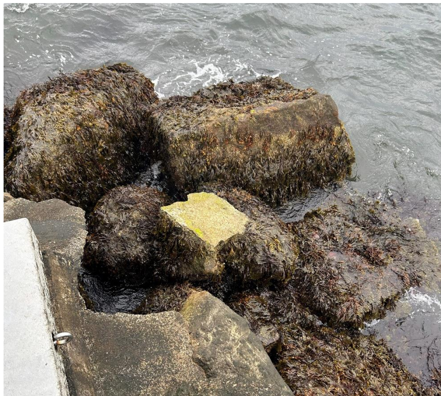
Photo 14: Indianola steel pier shifted armor stones Southeast corner
