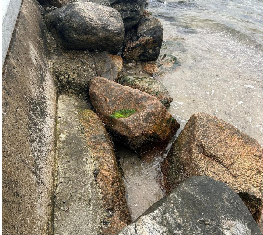
Photo 13: Indianola steel pier displaced armor stones South side
