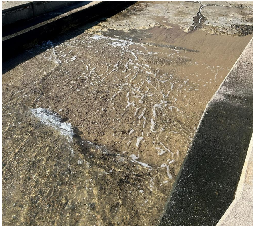
Photo 36: Sea View boat launch sand and stones collecting at ramp toe
