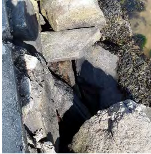
Gap in Armor Stone Revetment Requiring New Stone Infill
