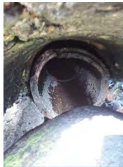
Broken Last Section of Pipe
