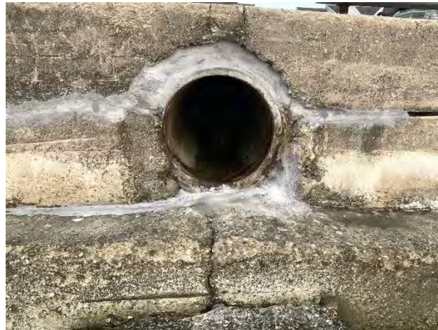
Image 15: Drain outfall (Blue Heron Way, 2023)
