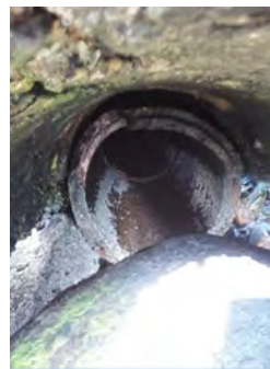
Broken Last Section of Pipe
